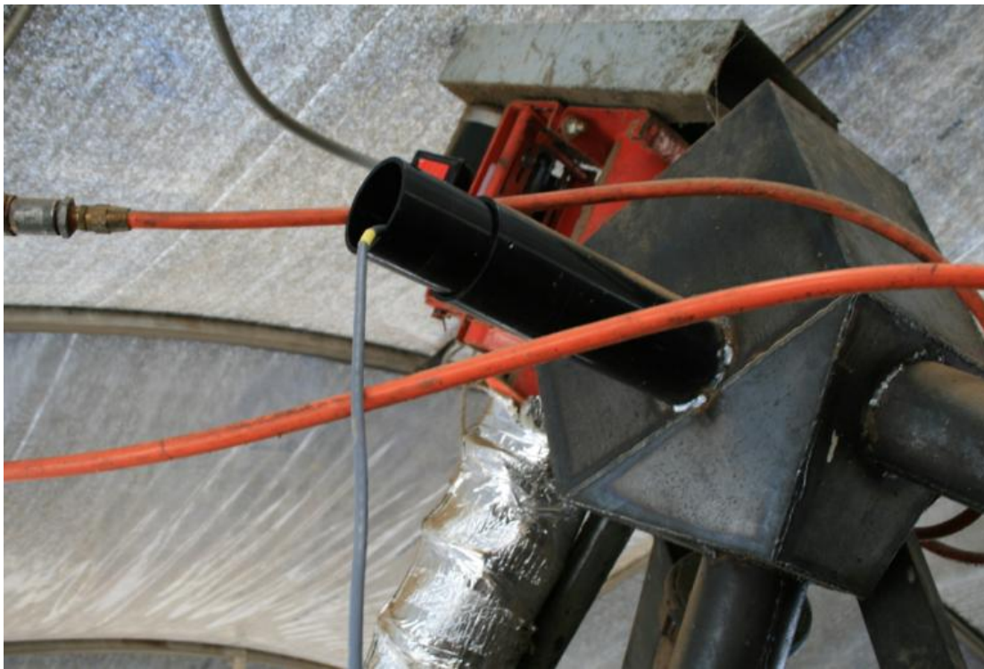
Figure 13 – Installation of the sensor in the seed stream – outside seed hopper.
